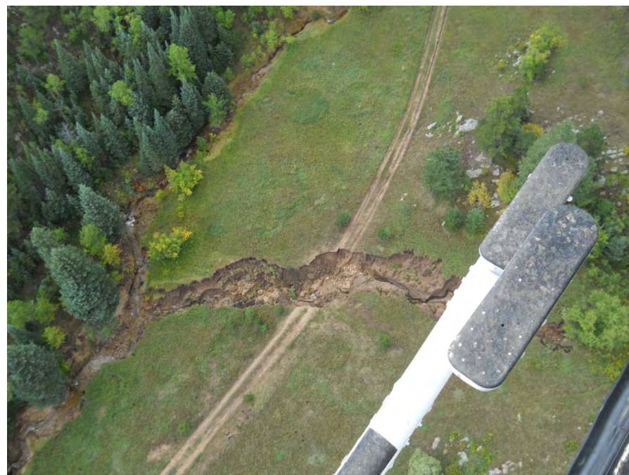
Above: Forest road impassible and in need of redesigned stream crossing to accommodate higher water volume
